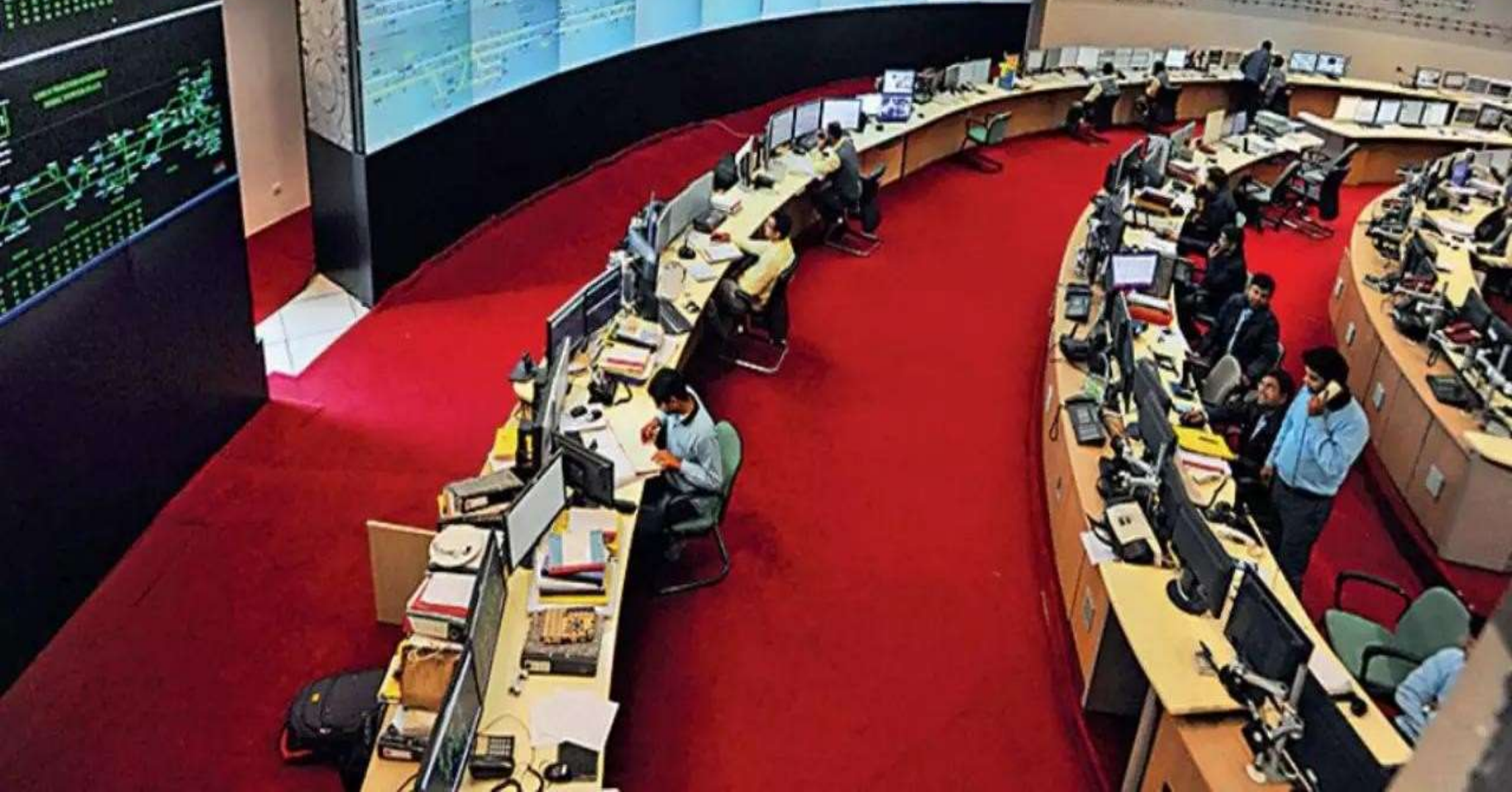
DELHI METRO BARAKHAMBA ROAD OCC
